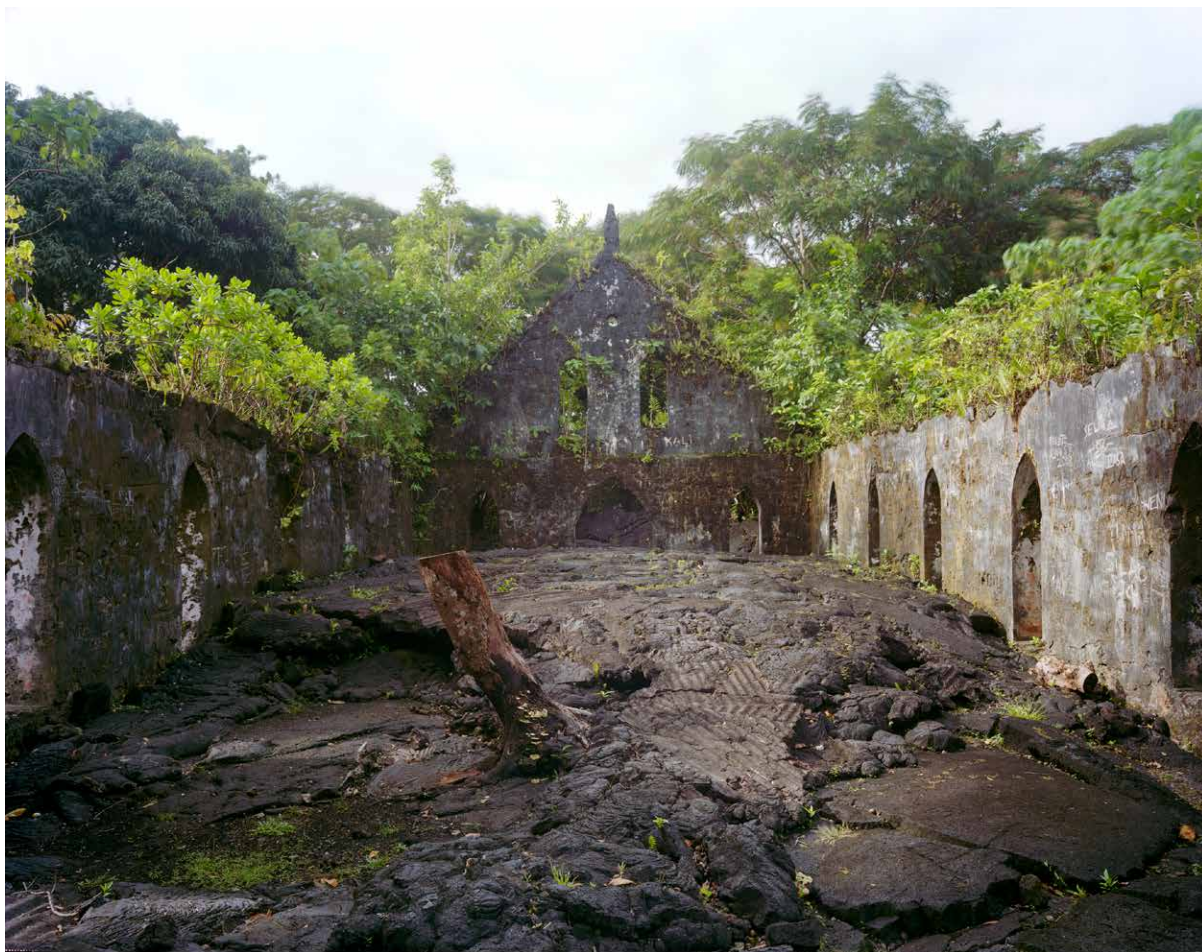
5.6. 18 July 2008. Interior of a London Missionary Society church overwhelmed by lava in 1905. Saleaula, Savai'i, Samoa.
