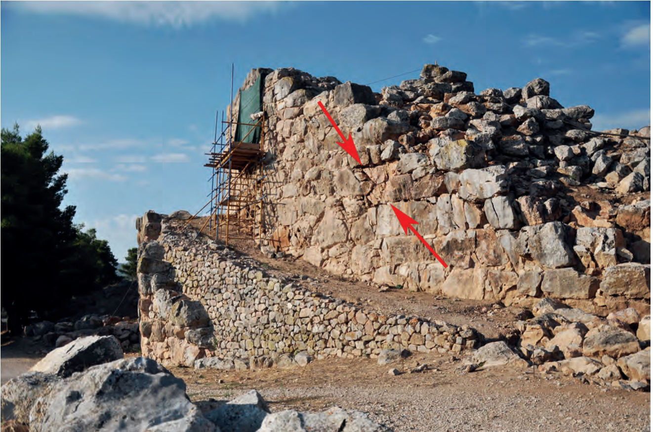
Figure 4 Tiryns east side of citadel, main entrance with Great Ramp showing badly flaked lithofacies E blocks
